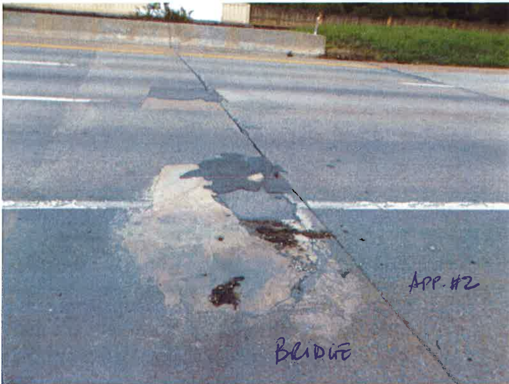
Pic # 31 Patches at Abut. 2; Bridge No. 19-I440-4.17R
